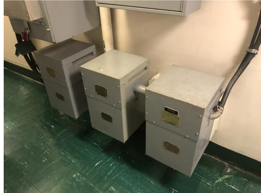
Transformer bank onboard CV-41 © 2024 by Norbert Doerry Licensed via CC BY 4.0
