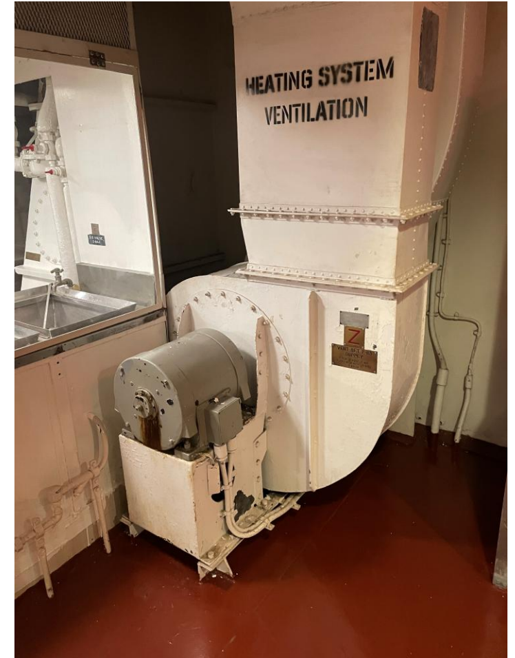
Ventilation Fan Motor © 2026 by Norbert Doerry Licensed via CC BY 4.0
